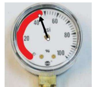
Insufficient dynamic pressure
